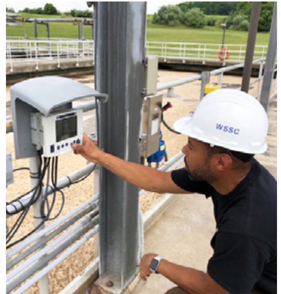
Greg Whitley at the Seneca WRRF using the IQ SensorNet system.
