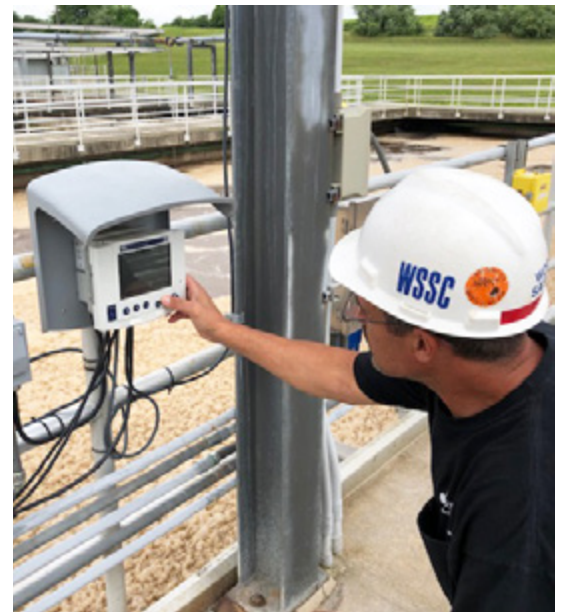
George Kosanovich checks an IQSN 2020 3G controller at the Seneca facility.
